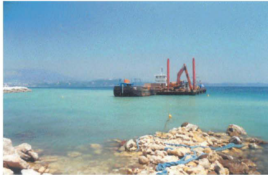
Fig. 72. . A barge and rock-clearing equipment during the digging of an access channel to a port in the Var (France). The turbidity of the water caused by the work is obvious. Photo by P. Bonhomme.
